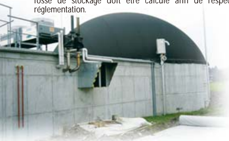
Photo 5 : Post-digester (source Aile)
